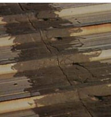
Seam and fastener problems.
