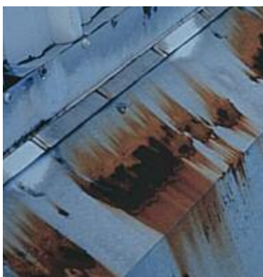
Rust and corrosion.
