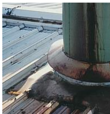
Cracks or leaks around penetrations.
